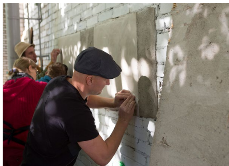
Estonia, Ecomess of the Centre of Sustainable Renovation and Partners 2014, Tallinn. Photo: Toomas Tuul, 21.09.2014
